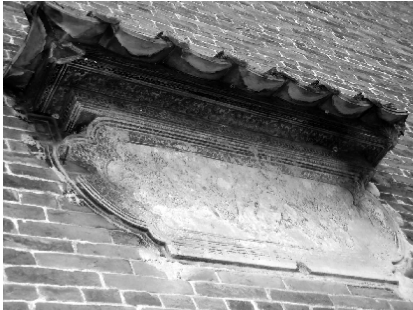
Figure 58. Plasterwork of Lintel of a portal in Zizheng Daifu ancestral temple in Huadu district of the city of Guangzhou (1863).
