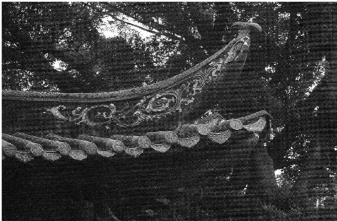
Figure 91. The fish-tail plasterwork on the hip ridge.
