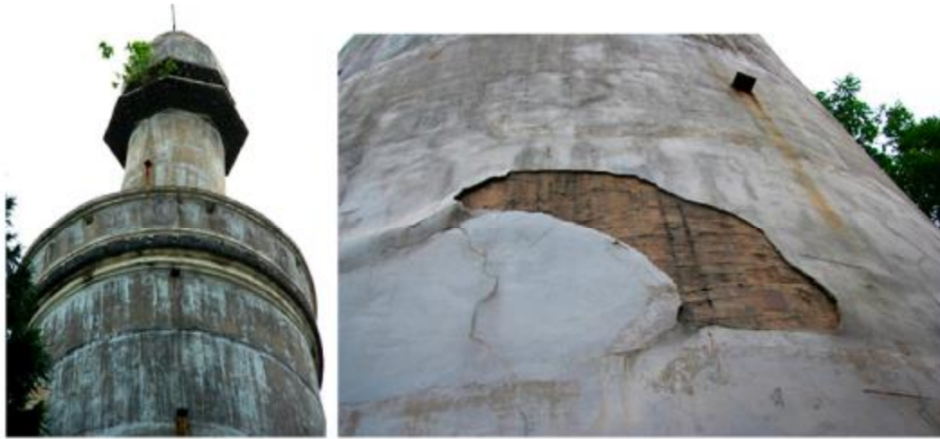
Figure 105. Part of tower body and decoration of oyster shell lime mortar on the surface.
