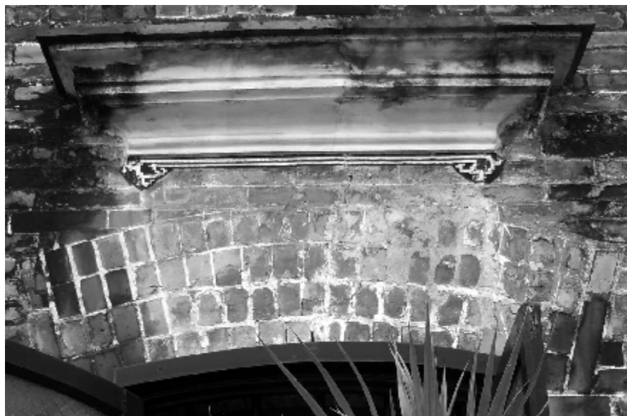
Figure 59. Decorative plaster of lintel of a window in back hall of Chen's Clan temple (1894).
