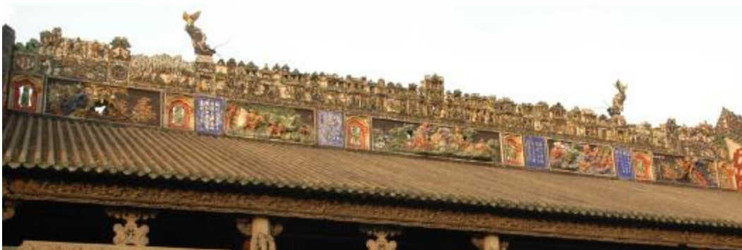
Figure 20. The decorative plasterwork on the main ridge of the roof in Juxian Hall of Chen Clan Ancestral Temple in 1894.
