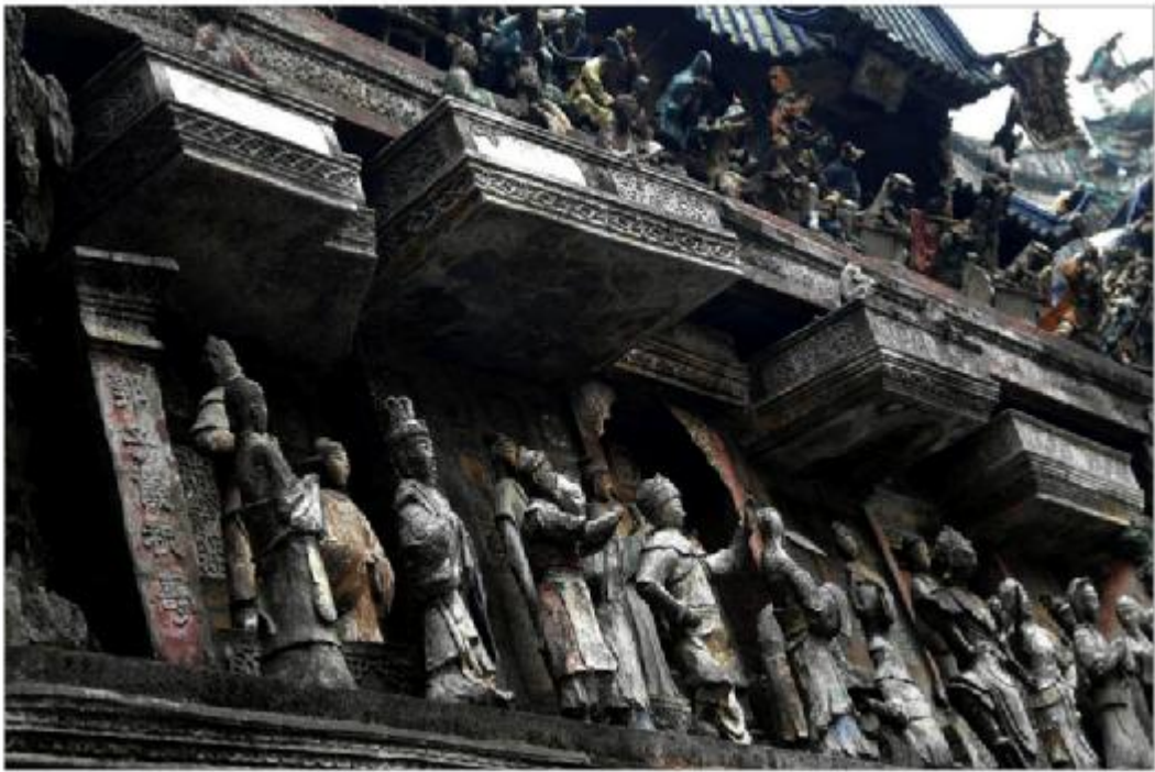
Figure 36. the decorative plasterwork 'congratulate on Guo Ziyi's Birthday' on the watching ridge in Xujiang Ancestral Temple about in 1871.
