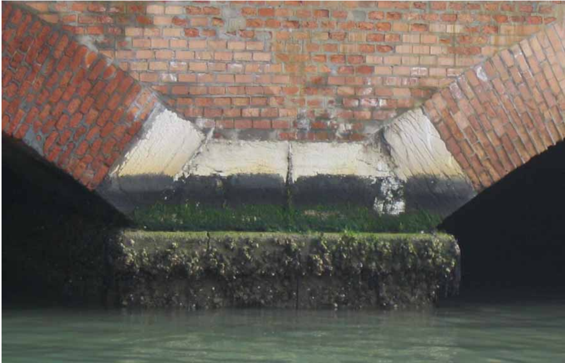
Fig 4.23 - The 219 th pier, it is possible to notice vegetation and biological attacks and stains.
