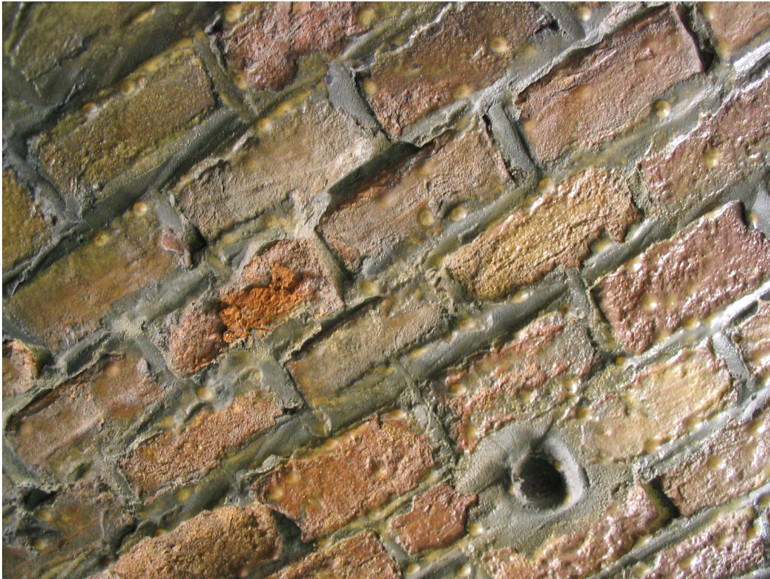
Fig 4.22 - Detail of the masonry of the vault, it is possible to notice one of the holes drilled for the injection carried out during the restoration and repointing..
