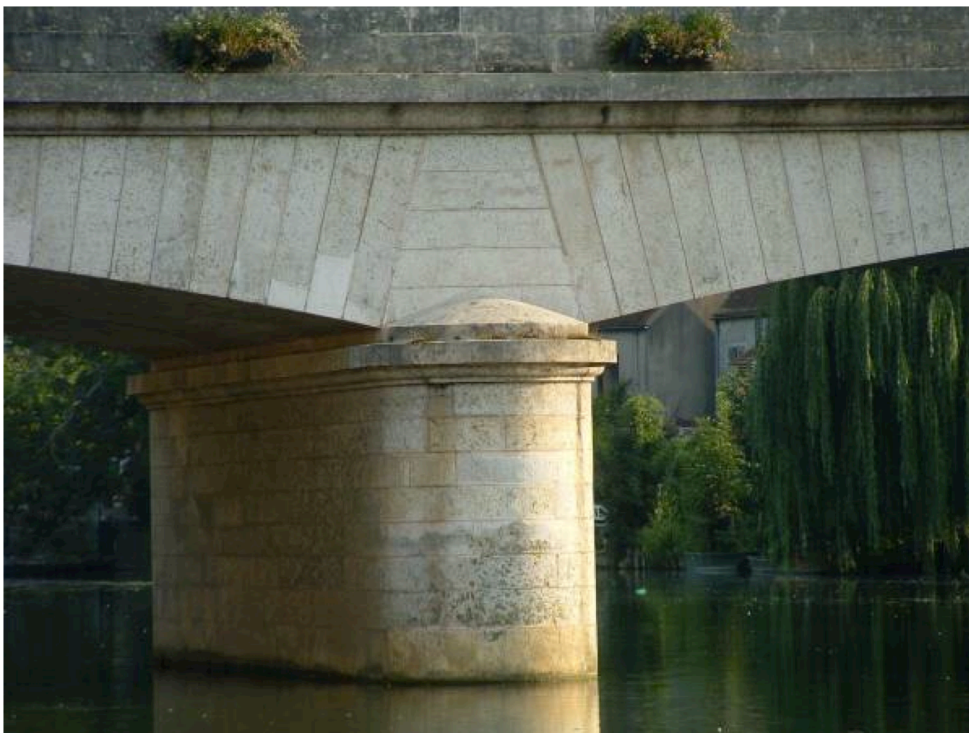
Fig 1.13 - Perronet, pont de Meumurs, detail of the connection between pier and arches.
