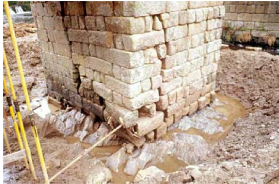
Fig 3.2 - Foundation and piers damaged because of scour
