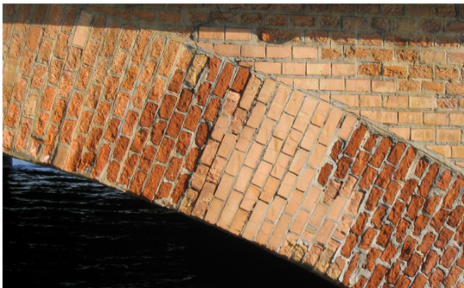
Fig. 4.9 - Particular of the masonry of one arch of the enlargement, it is possible to notice the substitution of blocks.
