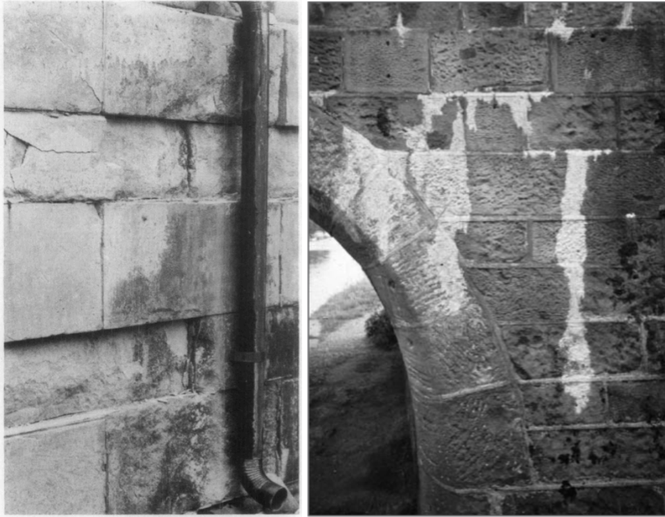
Fig 3.8 - Blistering (left) and leaching (right).
