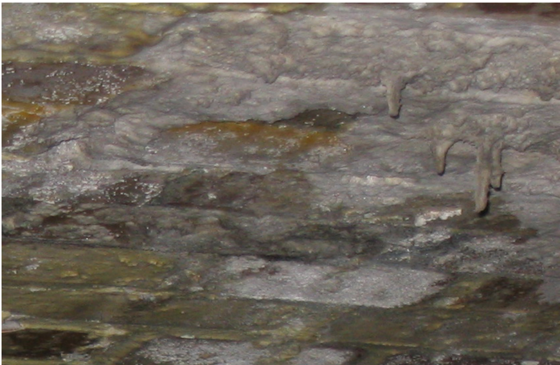
Fig 4.18 - Detail of the vault, calcareous crusts
