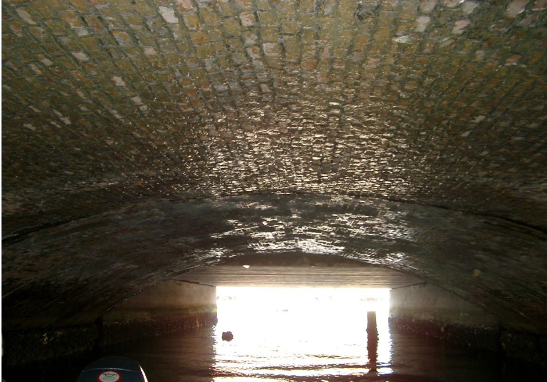
Fig 4.19 - View of the bridge from below, it is possible to notice the three bridge: the enlargement, the old rail-bridge, the new rail-bridge.
