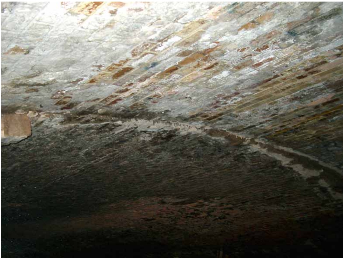
Fig 4.20 - Detail of the connection between the enlargement and the old rail-bridge, it is possible to notice diffused salt attack, leaching and dislocation of material.
