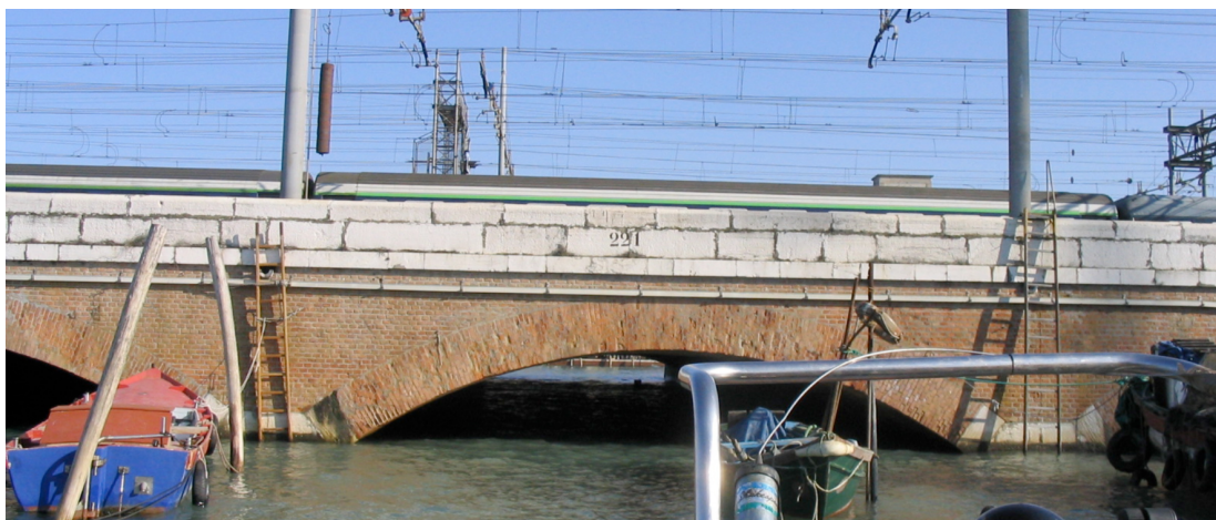
Fig 4.10 - Lateral view of the 221 st arch, in the enlargement, it is possible to notice the masonry of spandrel walls and the railings in Istrian stone.
