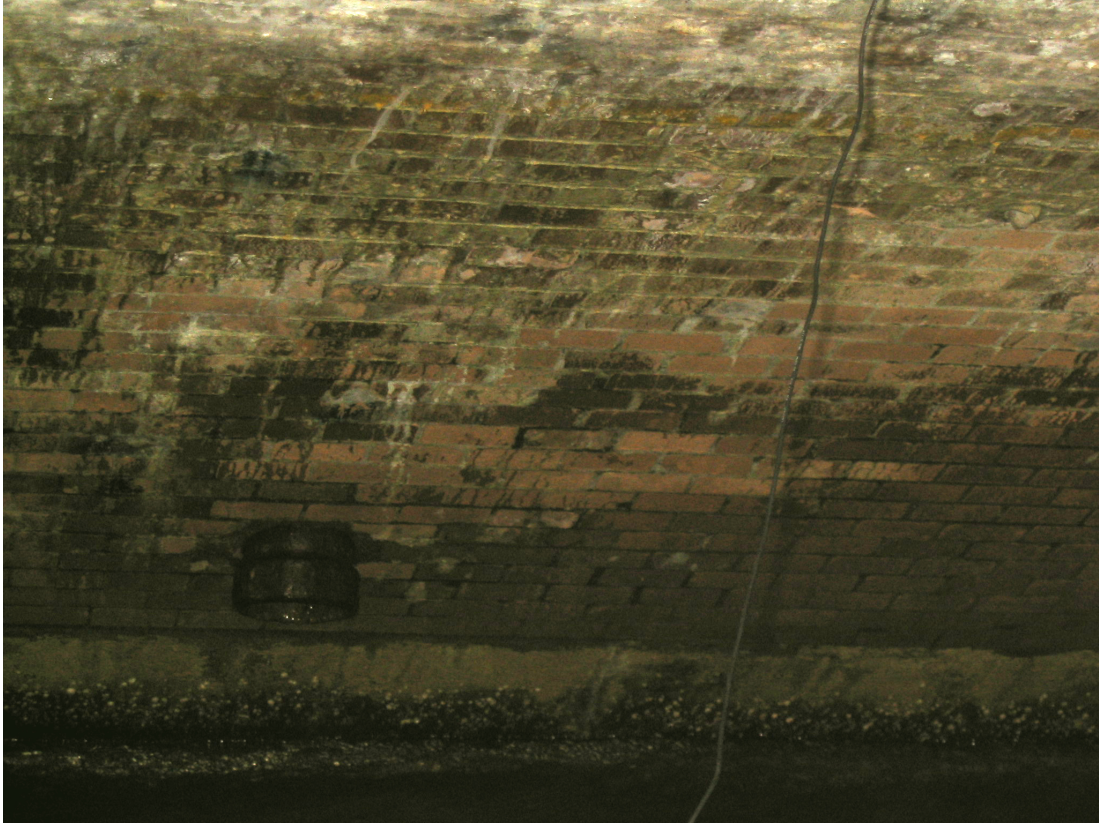
Fig 4.17 - View of the vault form below, it is possible to notice: the pipe of the waterproof system, leaching in the masonry of the barrel vault.
