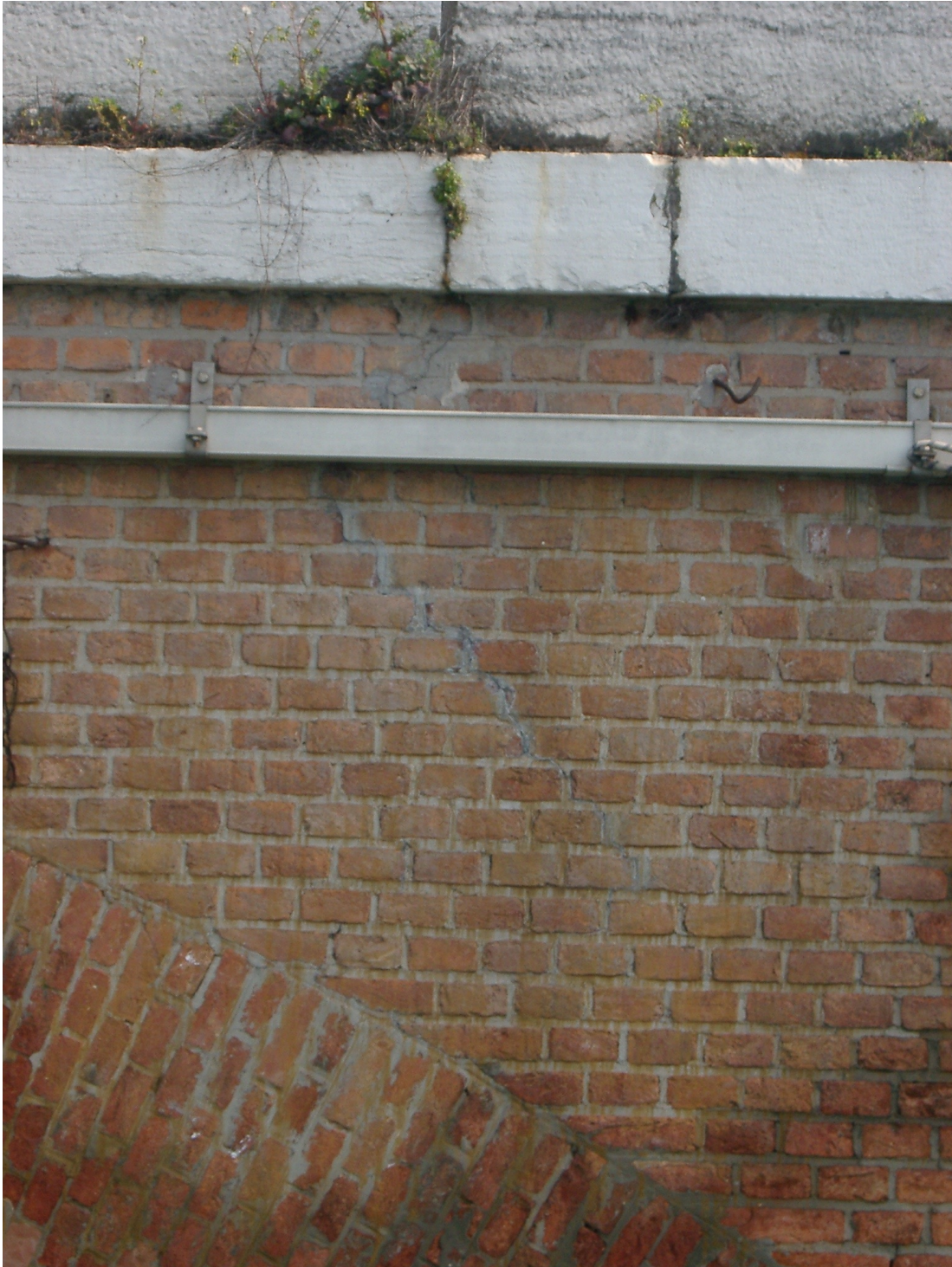
Fig 4.24 - Cracking in spandrel walls, vegetation in the railing.
