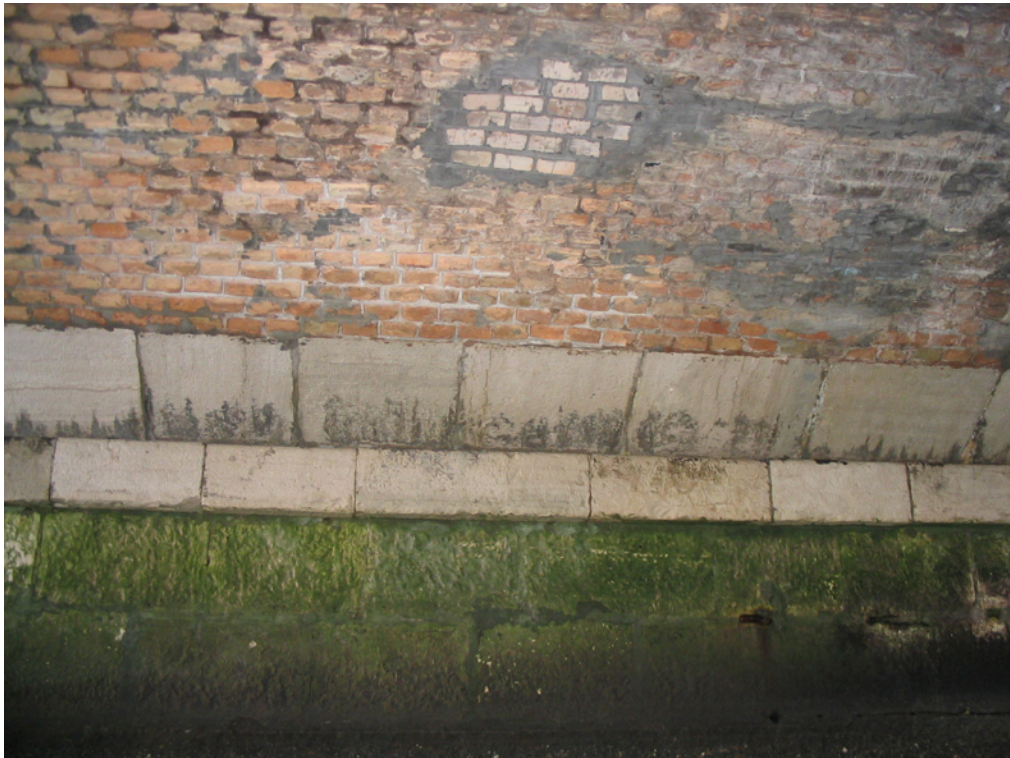
Fig 4.16 - Detail of the vault form below, it is possible to notice: un-correct intervention of substitution of block, use of cementitious mortar, biological and vegetation attacks in the pier
