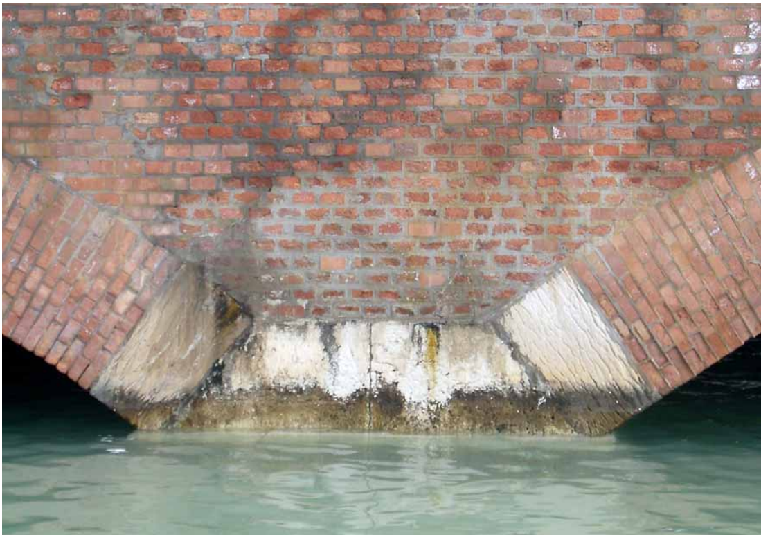
Fig 4.24 - The 220 th pier, it is possible to notice stain in the Istrian stone, substitution of blocks and repointing in the spandrel.
