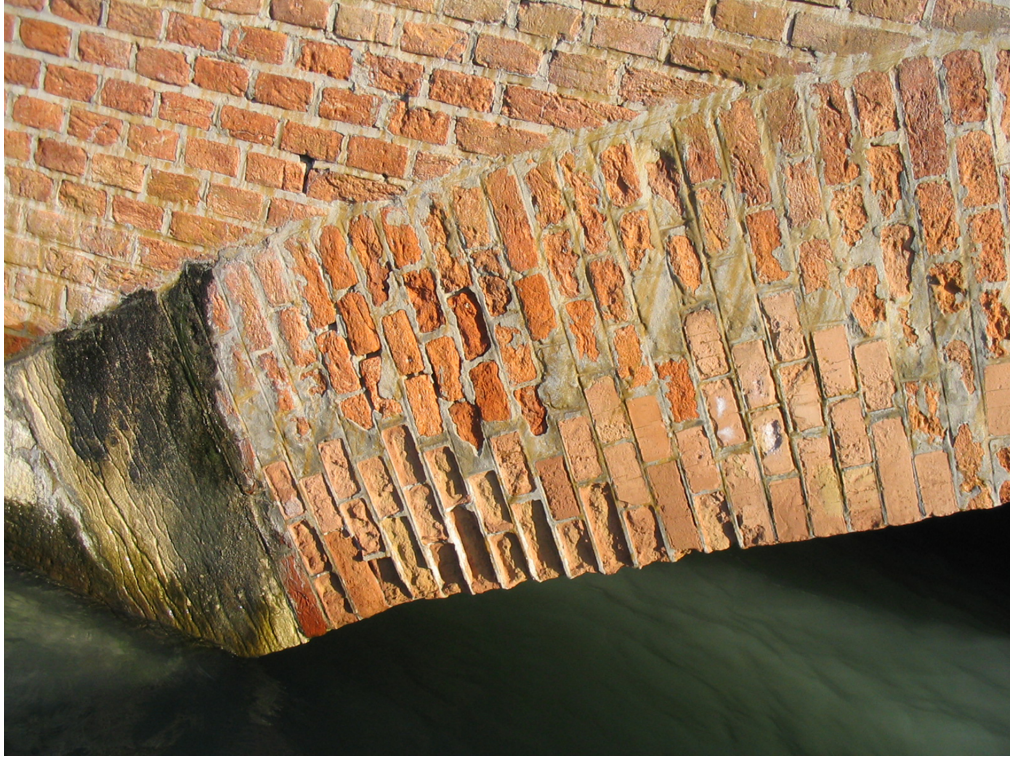
Fig 4.15 - Detail of springing of one arch, it is possible to notice: delamination of blocks, substitution of blocks and repointing carried out with heavy mortar; the Istrian stone shows is stained at the height of tides.
