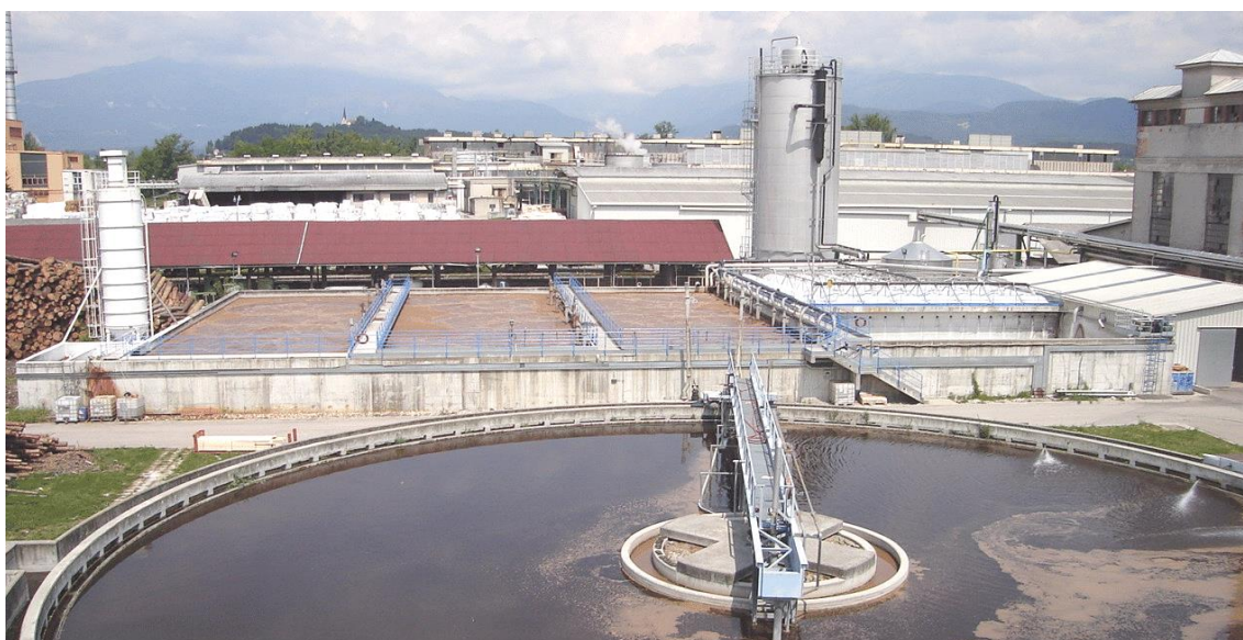
Figure 7. Wastewater-treatment plant in Količevo Karton with the secondary-sedimentation tank in the front.
