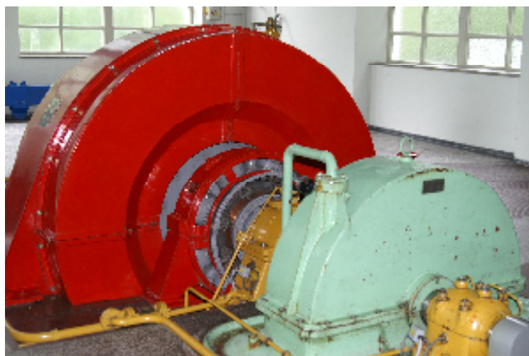
Slika 3.3 Generator v HE Savica (2007)
