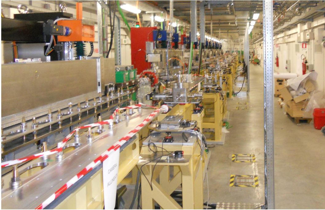
Figure 3.7: Undulator hall of FEL-1.
