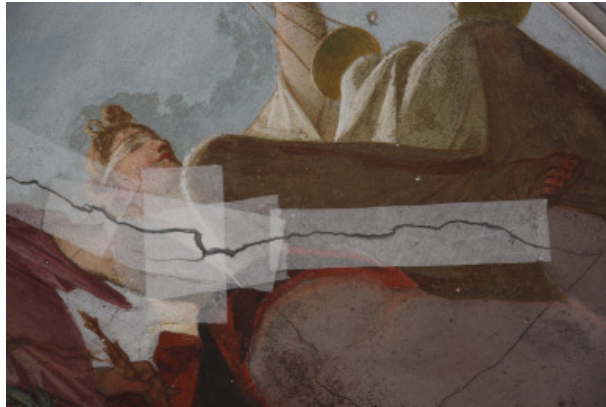
Image 76: Crack of false ceiling in the portego
