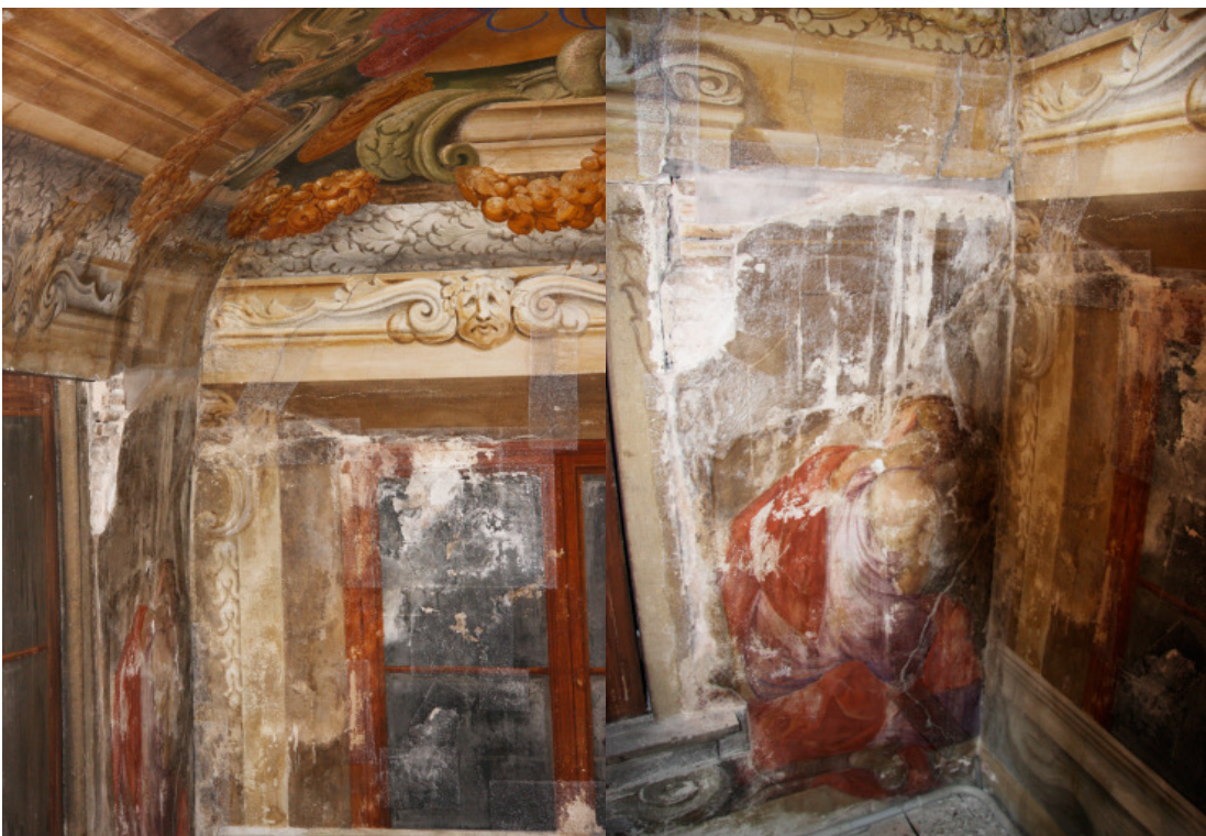
Image 100: Decay for seepages
