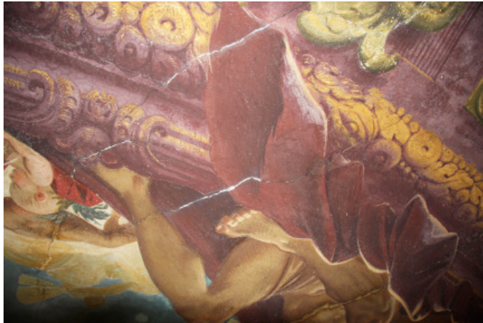
Image 96: Cracks of the false ceiling
