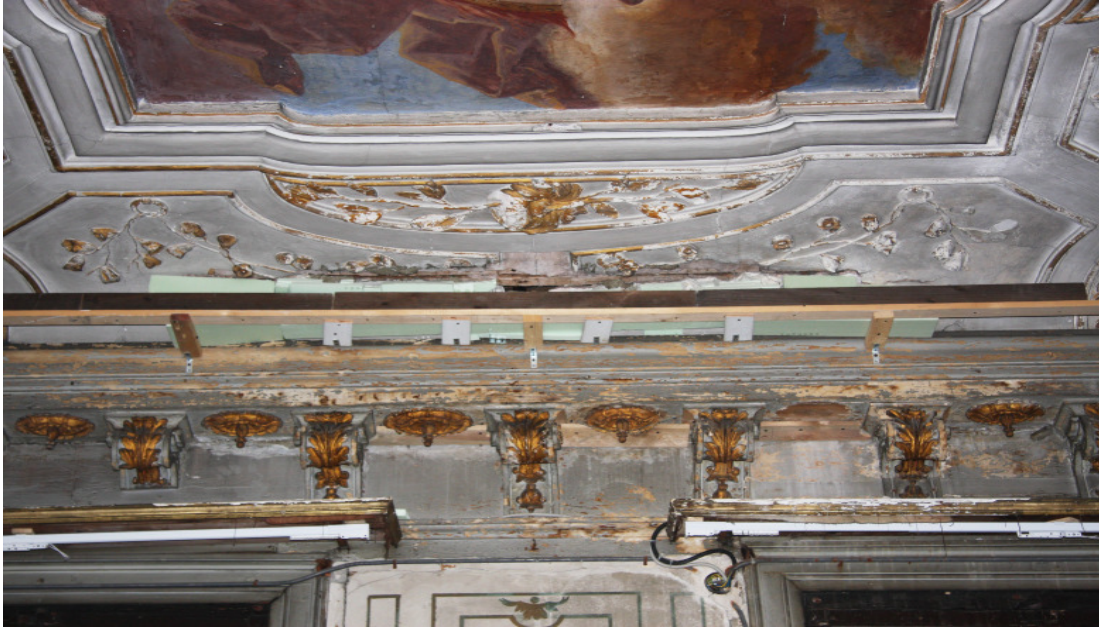
Image 78: Structural problem of the false ceiling in room A.19
