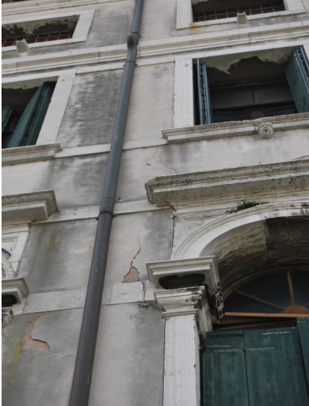
Image 89: Cracks of principal elevation
