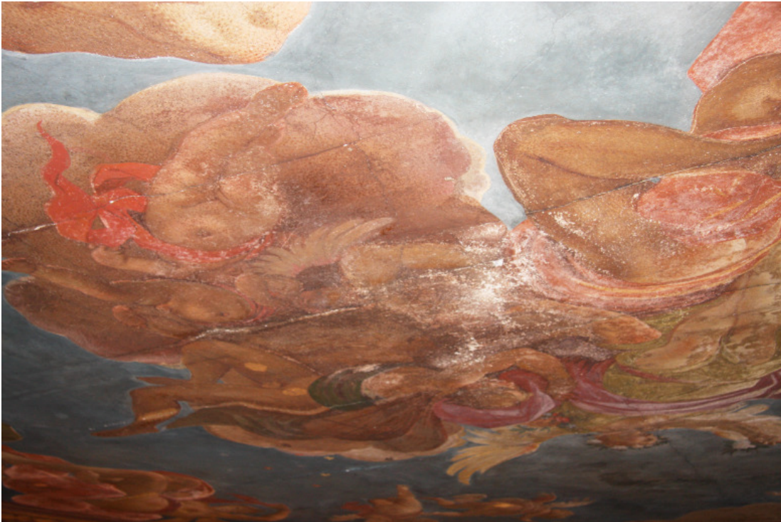
Image 99: Superficial erosion, cracks and lacuna
