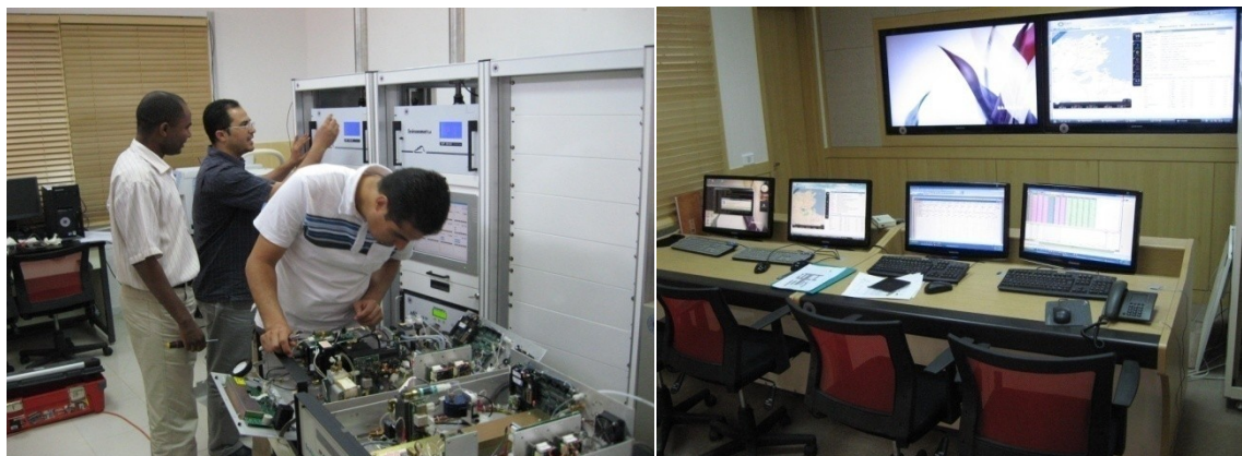
Figure 7. Information system and new supersite station installed in 2010 in Park Mourouj (Source: RNSQA)
