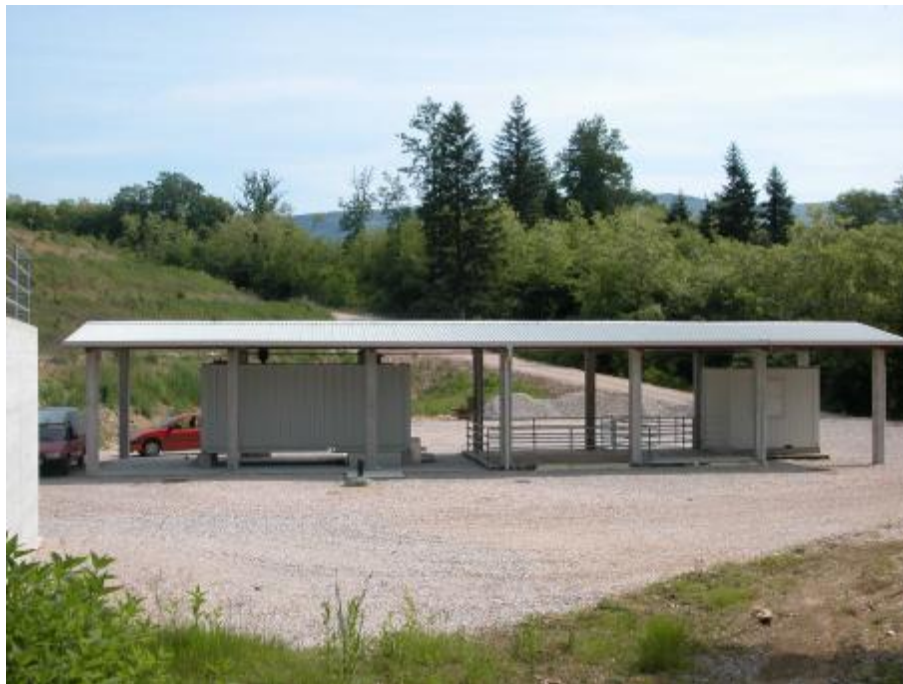
Figure 9: Reverse osmosis plant at Landfill Stara Gora. Source- photo Lucija Kobal, 2004.
