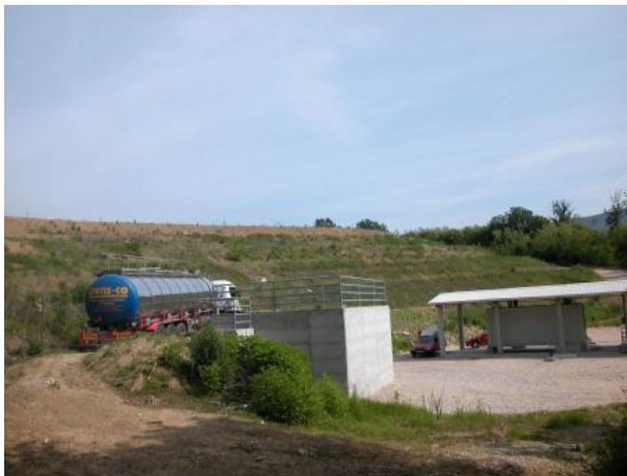
Figure 10: Emptying of tanker to reservoir of Reverse osmosis plant. Source- photo Lucija Kobal, 2004.
