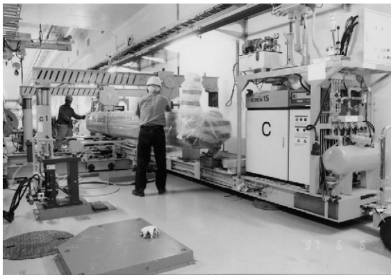
Fig. 6. A picture of a scene of magnet installation. A 6 m long HER-B magnet is handed over from the magnet transporter to the movable table to be installed to assigned position.
